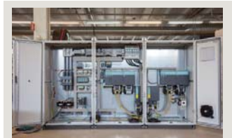
Electrical cabinets • EU and international standards applied
