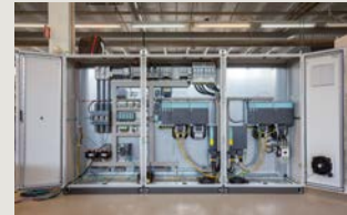
Electrical cabinets • EU and international standards apply
